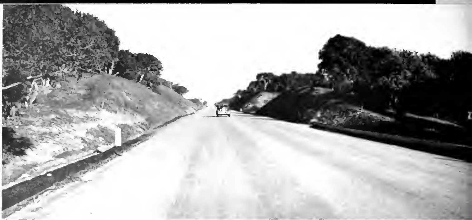
View of unfinished realigned section of Prunedale-Castroville road showing straight tangent eliminating many curves and grade
